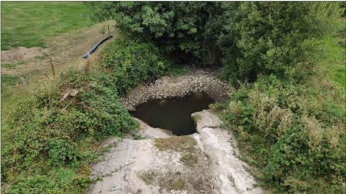
Plate 4.2 Example of a natural and artificial barrier to fish passage on the karstic Owveg River at Spink Bridge (site B7), where the river frequently runs dry over an excessively high & fractured bridge apron
