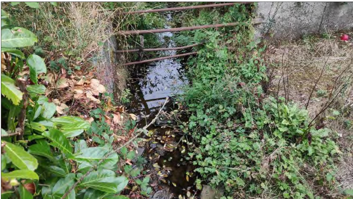
Plate 4.25 Representative image of site B9 on the Graiguenahown Stream, September 2022 (downstream of twin pipe culvert)
