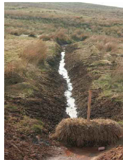
STRAW BALE TEMPORARY SILT TRAP (FROM WIND FARM CONSTRUCTION GOOD PRACTICE GUIDE)
